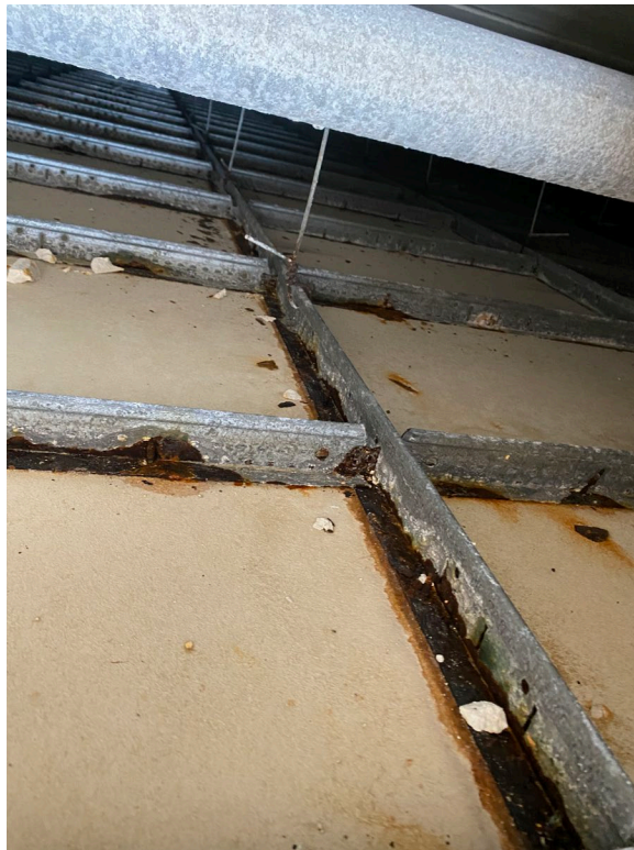
Picture 4: Typical corroded flanges of garage soffit attachment
